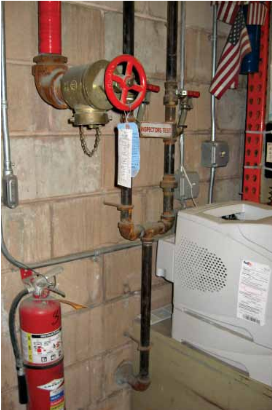
Best practices for fire protection are integrated through design, installation and beyond. A inspector's test location at the remote end of a system would follow best practice protocol.
